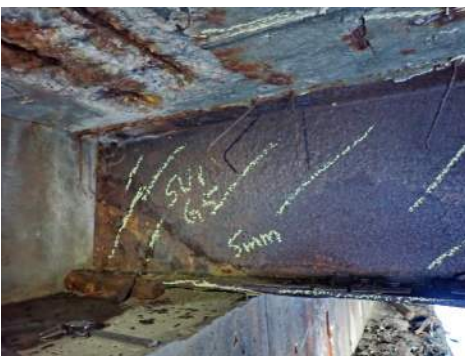
G5 at SU1. Note: Typical corrosion.
