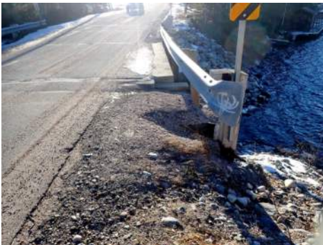
Approach - Wearing surface - NE. Note: Erosion starting to encroach roadway
