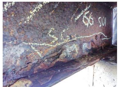
G6 at SU1. Note: Typical corrosion.
