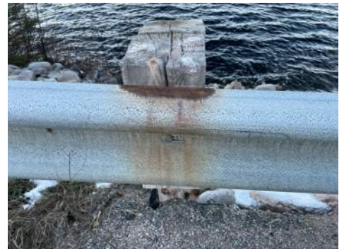
Coatings - Railing. Note: Typical rusting.
