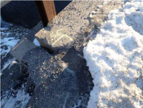
Deck top - SE. Note: Spall repaired with asphalt.
