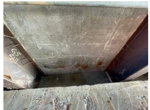
Deck Soffit - Interior - SU1 between G4/G5. Note: Typical delamination and rust staining.
