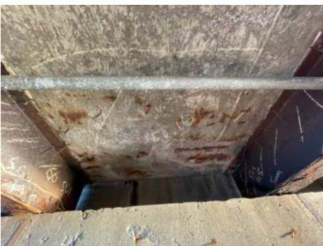
Deck Soffit - Interior - SU1 between G5/G6. Note: Typical spalls with exposed rebar, delamination and rust
