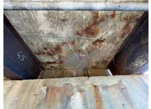
Deck Soffit - Interior - SU2 between G5/G6. Note: Typical spalls with exposed rebar, delamination and rust
