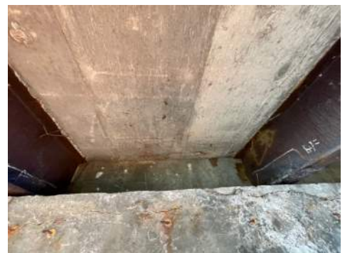
Deck Soffit - Interior - SU2 between G2/G3. Note: Typical spalls, delamination and rust staining.
