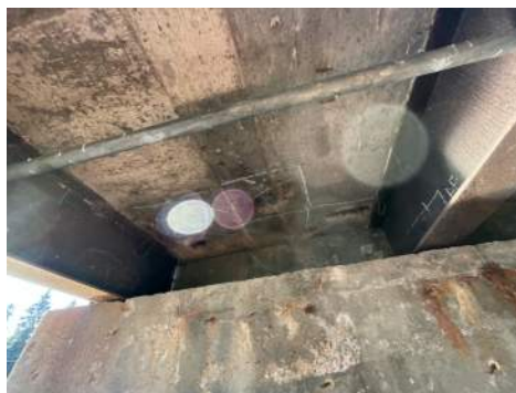
Deck Soffit - Interior - SU2 between G1/G2. Note: Typical spalls with exposed rebar, delamination and rust
