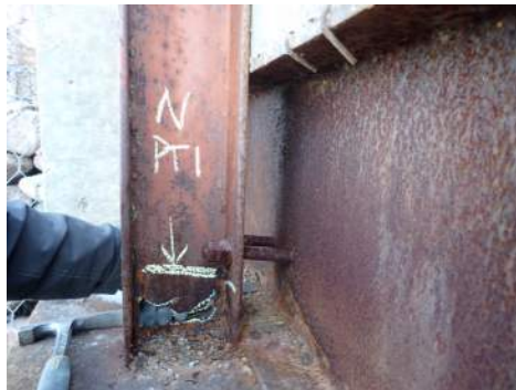
Posts - North PT1. Note: Corrosion hole through bottom of web.
