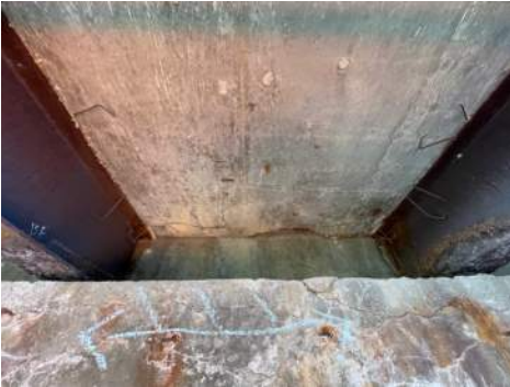
Deck Soffit - Interior - SU2 between G3/G4. Note: Typical spalls with exposed rebar, delamination and rust
