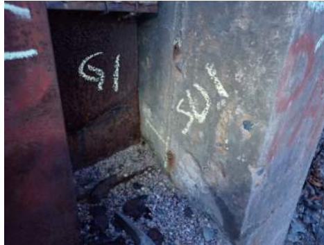
SU1 Ballast wall - at G1. Note: Mechanical spall behind bottom flange.
