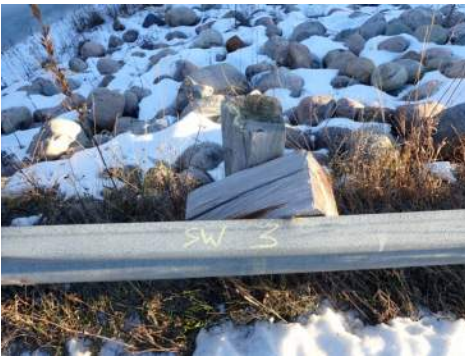
Posts - SW Approach - PT3. Note: Rotated blocking and section loss on post.
