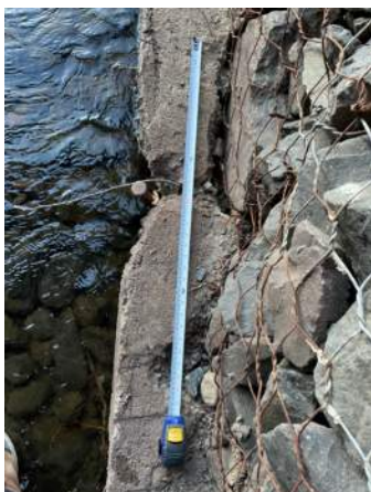
SU1 Abutment Wall - Footing. Note: Typical crack and spalls.
