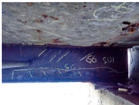
G6 at SU1. Note: Typical corrosion.
