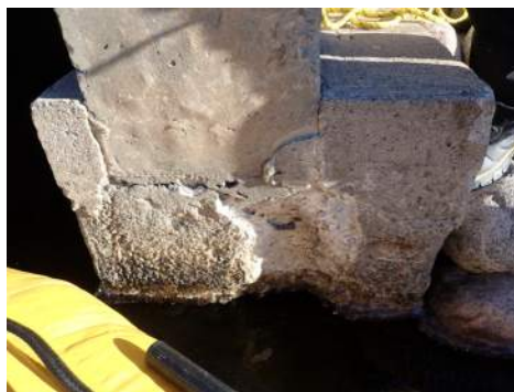
Inlet - SW corner. Note: Disintegration of footing
