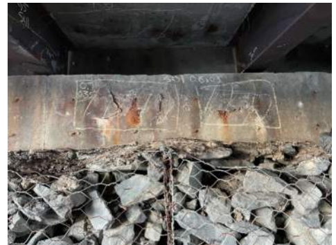
SU1 Abutment Wall. Note: Typical delamination, efflorescence and rust staining.
