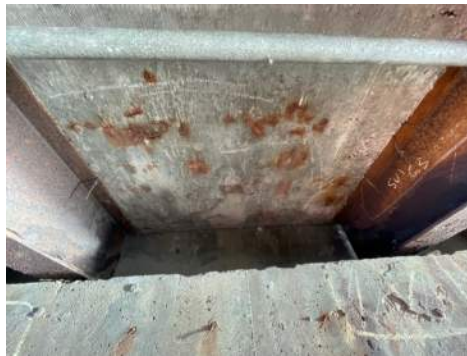
Deck Soffit - Interior - SU1 between G3/G4. Note: Typical delamination and rust staining.
