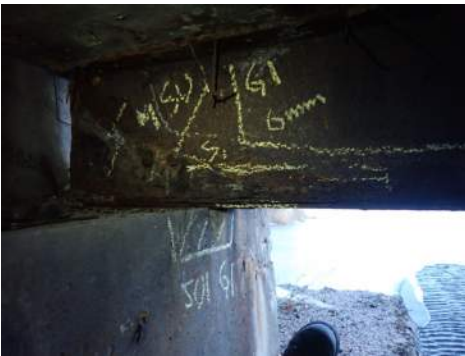
G1 at SU1. Note: Typical corrosion and spall below girder.
