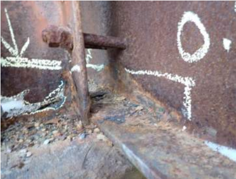
G6 at SU1. Note: Corrosion on web.
