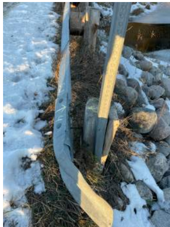
Posts - SW Approach - PT4. Note: Missing timber blocking.
