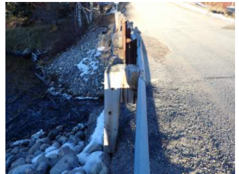
Posts - NW Approach - PT1. Note: Typical bottom of post is moving out due to loss of embankment material.
