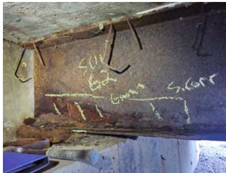
G2 at SU1. Note: Typical corrosion.
