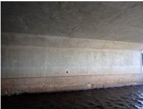
Culvert - South wall. Note: HL-M vertical cracks near Inlet.
