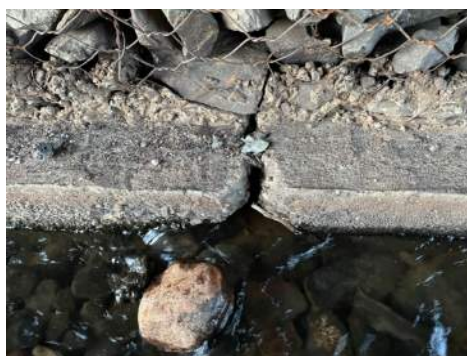
SU1 Abutment Wall - Footing. Note: Wide crack.
