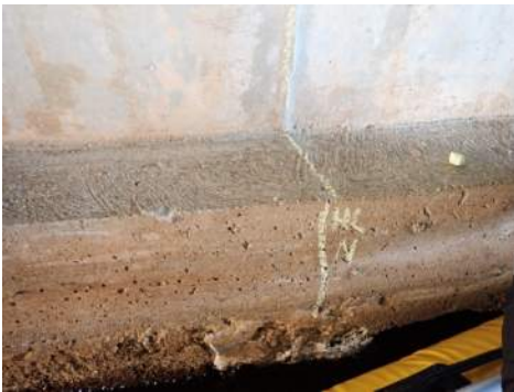
Footing - South wall. Note: Hairline to narrow crack extending from culvert into footing.
