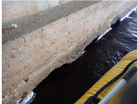
Footing - South wall near midspan. Note: Typical disintegration and exposed rebar
