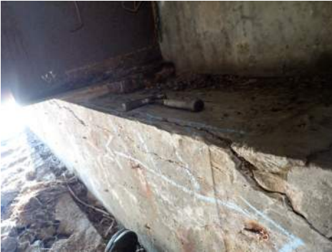
SU2 Abutment wall - between G3/G4. Note typical delamination, efflorescence and rust staining.
