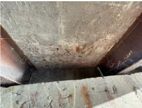
Deck Soffit - Interior - SU1 between G2/G3. Note: Typical honeycombing, delamination and rust staining.
