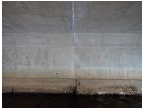
Culvert - North wall - mid-span. Note: Hairline to medium crack
