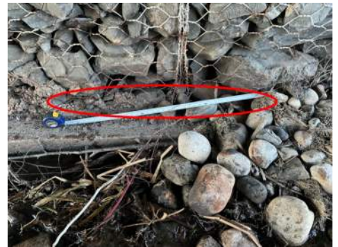
Slope Protection - SU1. Note: Typical holes in gabion wires.
