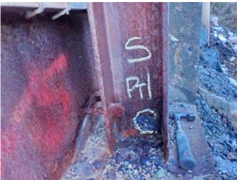
Posts - South PT1. Note: Corrosion hole through bottom of web.
