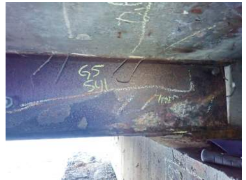
G5 at SU1. Note: Typical corrosion.
