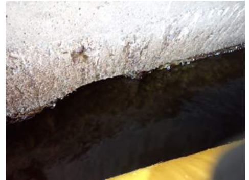
Footing - South wall. Note: Typical disintegration with exposed rebar.
