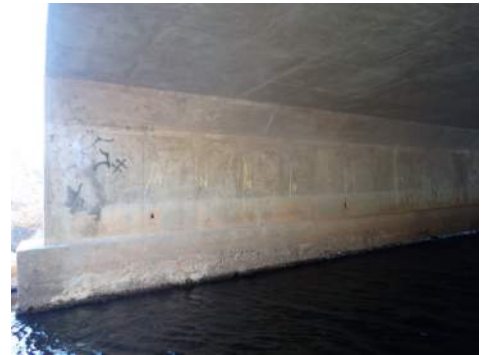
Culvert - South wall. Note: Typical HL-N cracks.
