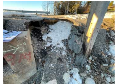
Approach - Wearing surface - SE. Note: Erosion trough encroaching roadway
