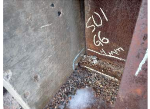
SU1 Ballast wall - at G6. Note: Mechanical spall behind bottom flange.
