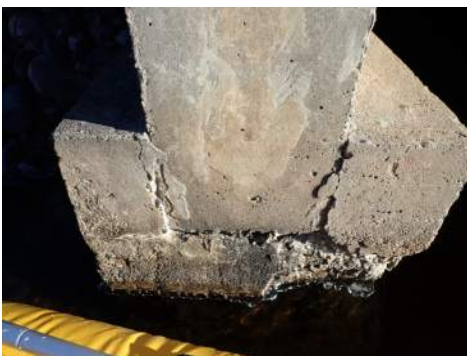
Inlet - NW corner. Note: Disintegration of footing
