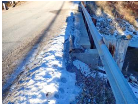
Approach - Wearing surface - SW. Note: Erosion trough encroaching roadway
