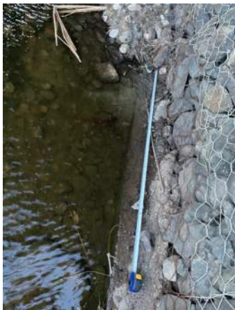
Slope Protection - SU1. Note: Typical holes in gabion wires.
