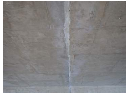
Culvert soffit - mid-span. Note: Hairline to medium crack
