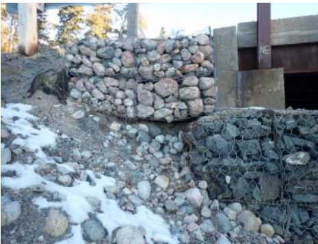
Embankments - NE. Note: Erosion under gabions.
