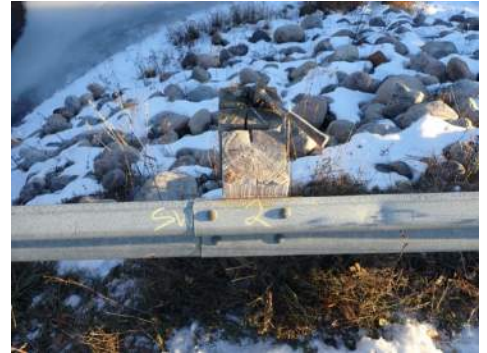
Posts - SW Approach - PT2. Note: Rot on top face.
