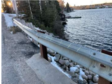
Railing Systems - NW. Note: Permanent deformation.
